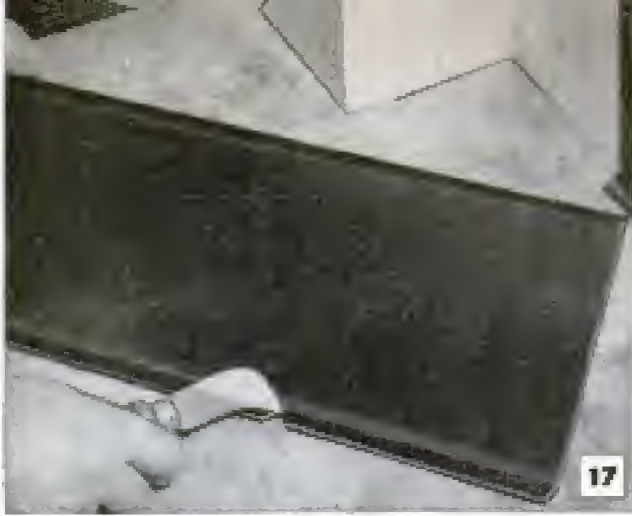
Above, asphalt tile used for top-set cove is notched, heated and bent to form inside corner as shown below
